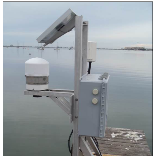
Clam Bayou site enclosure containing WaterLOG Radar and H-3553T Bubbler sensors.
